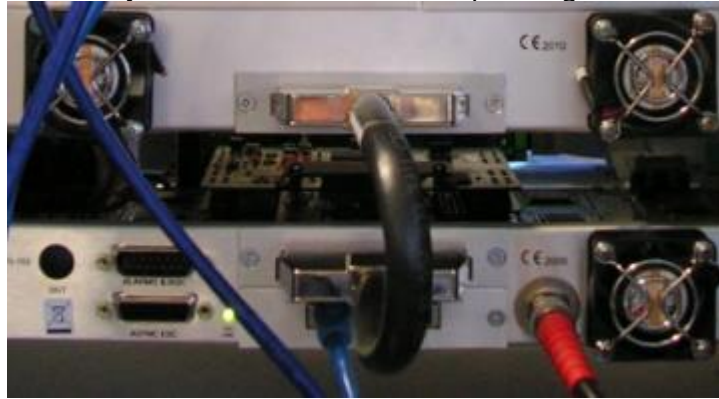
Figure 7-4 M3482 Umbilical Cable Connecting Switch to Backup Modem
