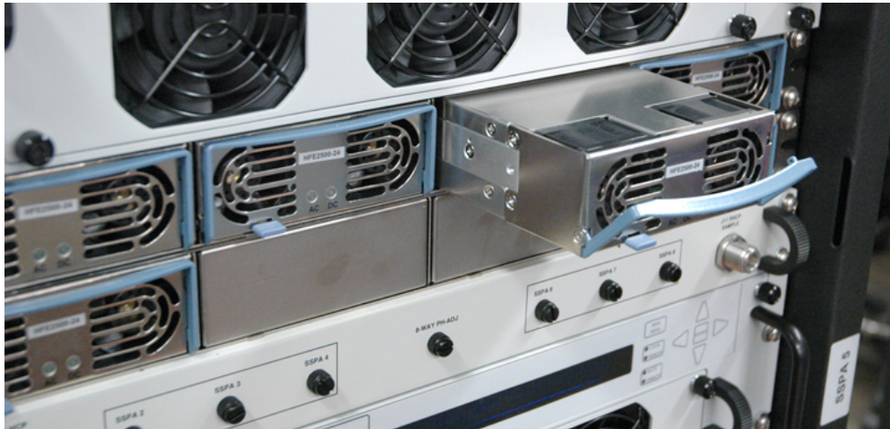
Figure 24: N+1 Power Supply
