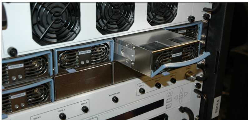
Figure 9: Install Power Supply Modules
