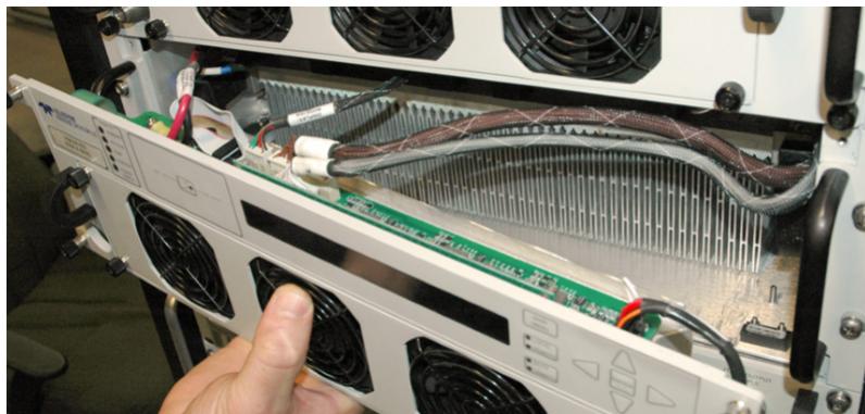
Figure 14: Tuck Cables into Enclosure and Re-seat Front Panel
