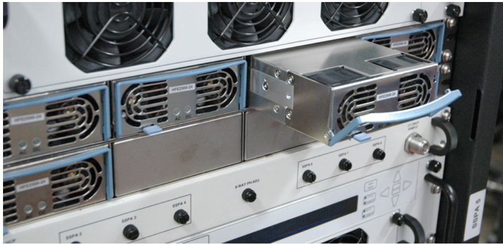
Figure 6: N+1 Power Supply
