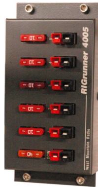
Figure 27: DC Distribution Panel
