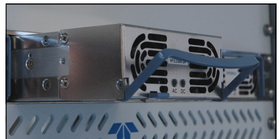
Power Supply Module in Chassis
