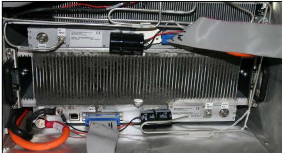
Figure 4-11: Example of Dust Blocking Heatsink Fins
