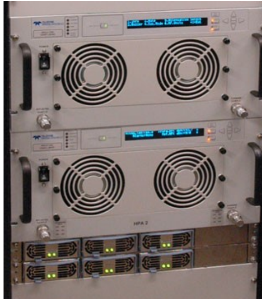
C-Band 1:1 Redundant System in the 5RU chassis, with N+1 redundant power supplies
