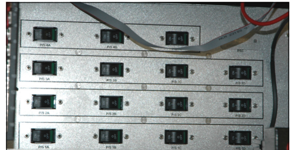
Circuit Breaker Panel
